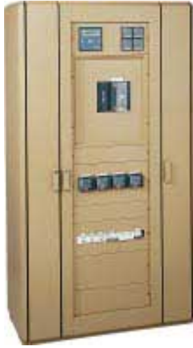
Digipact PM100 power meter and CLS150 indication and local control module on the front panel of the switchboard.
