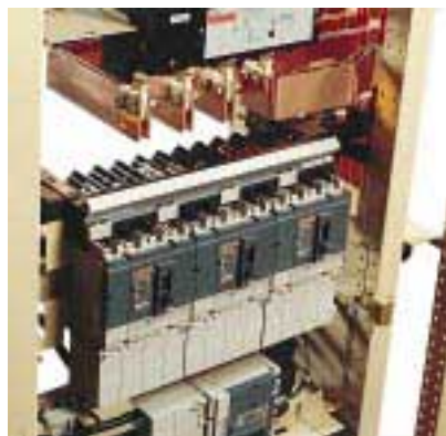
The auxiliary wiring is run in trunking.
