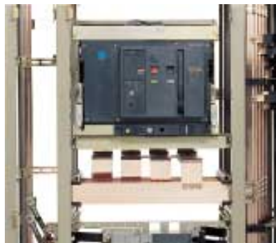
Masterpact 1600 A circuit breaker connected to Linergy busbars in a Prisma P cubicle, 600 mm depth
