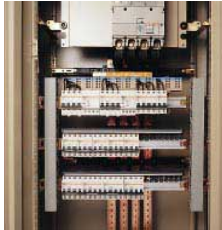
Connection via comb busbars and Multiclip distribution block.
