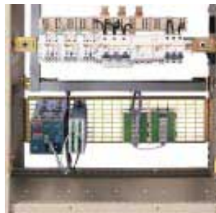
Digipact DC150 data concentrator and SC150 indication and control interface SC150 mounted on a slotted plate at the rear of the switchboard.
